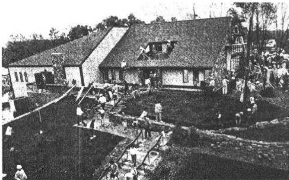
Forty-eight hours later, the 16,000-sq-ft Kingdom Hall in Waterbury, Conn., was almost complete.
